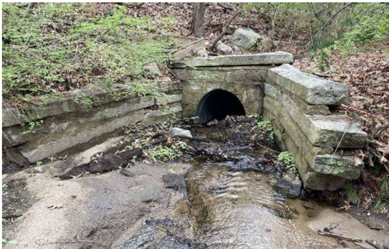
Figure 8. The inlet to the longest piped section of McQuesten Brook. The pipe is set 1-2 feet below the current bed elevation and drives incision in the reach upstream.
